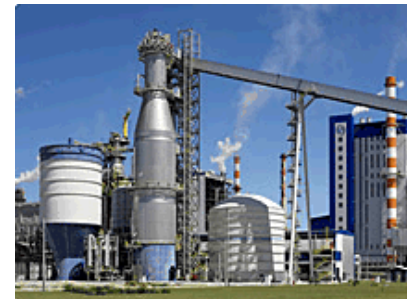
The continuous cooking plant, the heart of any paper and pulp plant. This one is from Metso.
